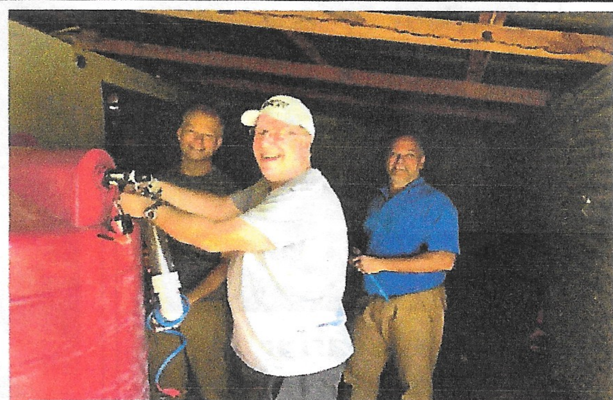
Team in Le Digue Mathiou, Haiti (above) Cistern and 2-tank system at Gros Morne, Haiti (below)
